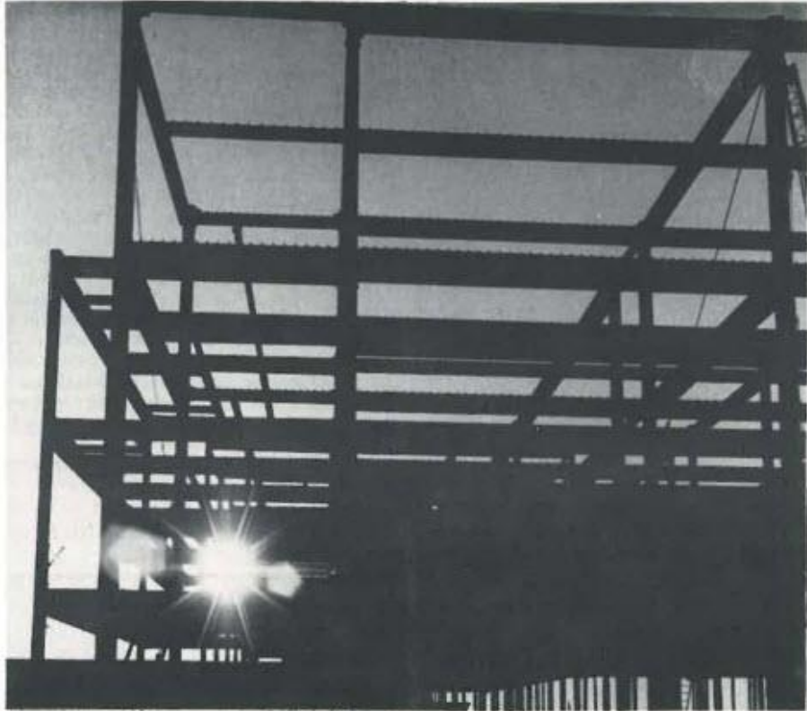
Arising from the red clay at the corner of Main and Devine Streets is the enormous new Law Center. The superstructure is almost in place and gives the illusion of dwarfing the Coliseum and the Sheraton Hotel. Occupancy of the building should be completed by September 1973.
